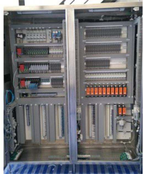
Inside of Control Panel
