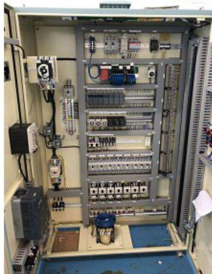
Inside of Control Panel
