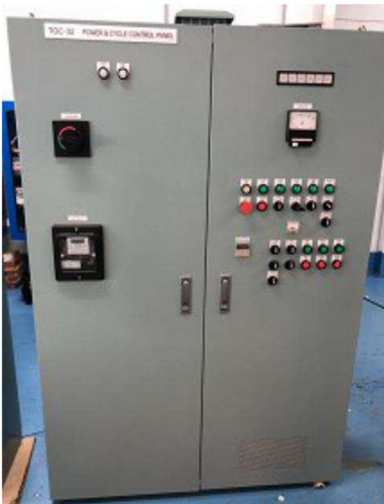
Control panel for Heat treatment factory
