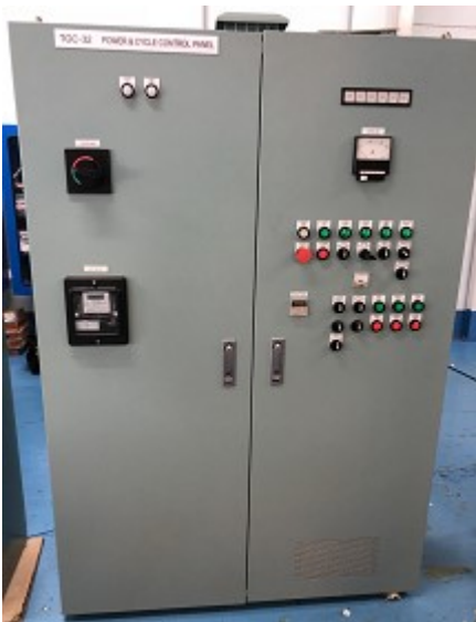
Control panel for Heat treatment factory
