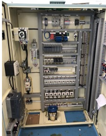
Inside of Control Panel
