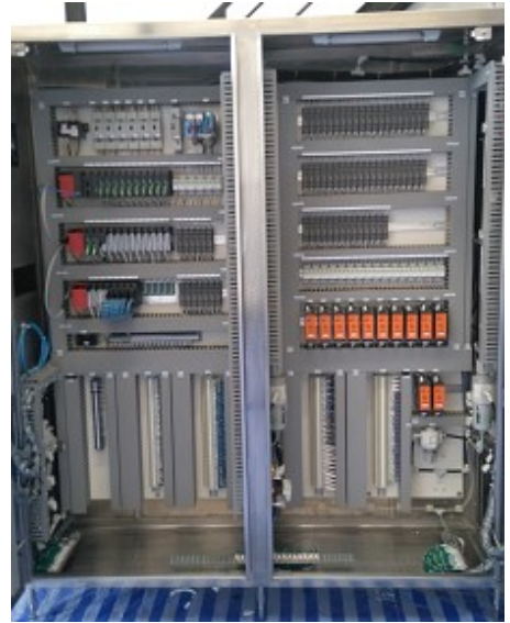
Inside of Control Panel
