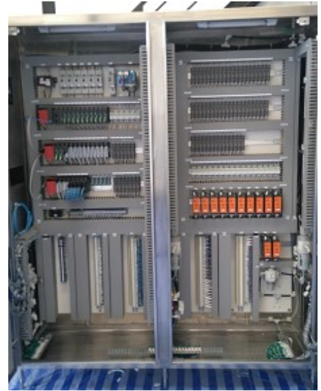
Inside of Control Panel
