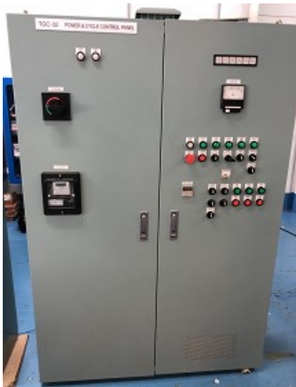
Control panel for Heat treatment factory
